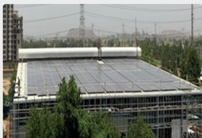
Solar panels at Bhiwadi site
